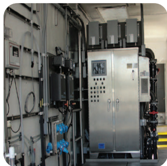
Controls and monitoring equipment
