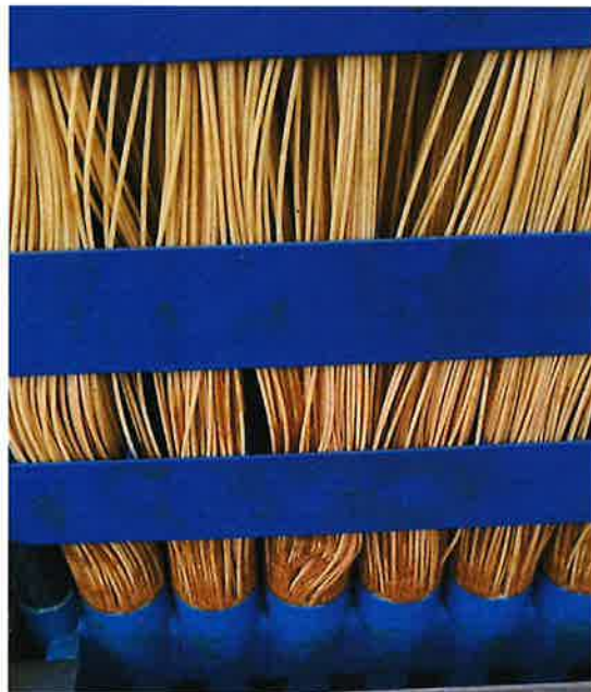
Figure 10. Module Showing Early Signs of Sludging
