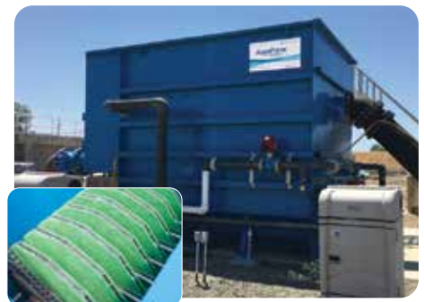
Linda County Water District, Olivehurst, CA
