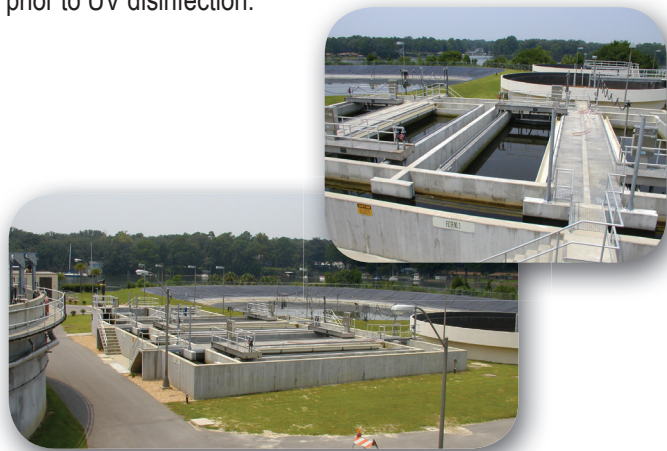
AquaABF® Filters at Millville WWTP
