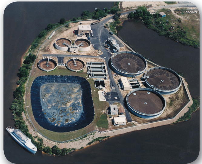
Millville's 3-basin AquaSBR ® system is shown on the right and the (4) AquaABF ® sand filters are shown adjacent to the post aeration basins.
