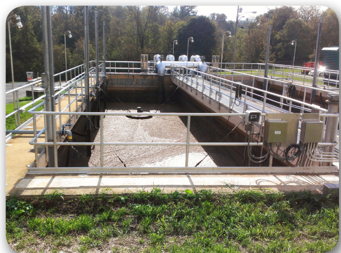
The biological treatment reactors of the Aqua-Aerobic® MBR.
