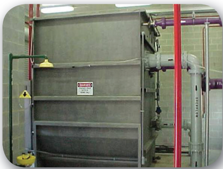
4-disk AquaDisk® filter located inside a small building at the York River Treatment Plant.
