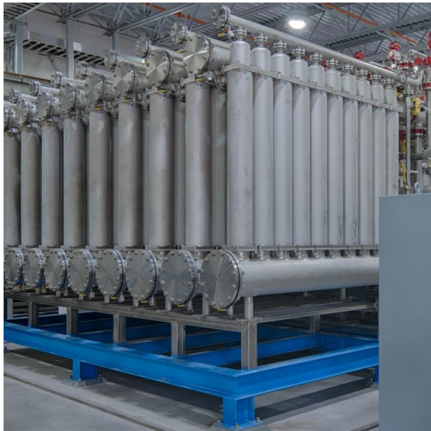
Figure 5 Primary Ceramic Membrane System Skid (One of Four)
