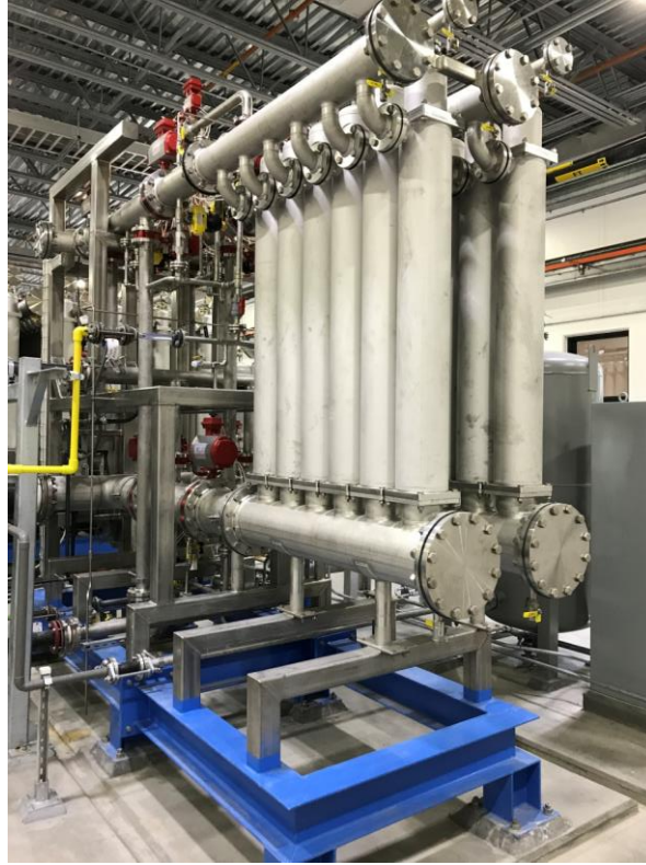
Figure 6 Backwash Recovery Ceramic Membrane System Skid
