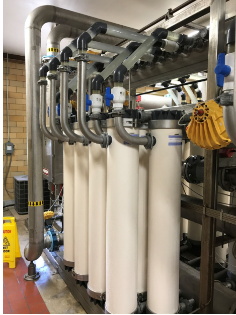
Figure 16. The New Two Rivers Modules with Rerouted Filtrate Piping
