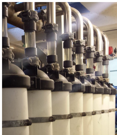
Figure 8. Original Butler Membrane Modules with Clear Filtrate Piping
