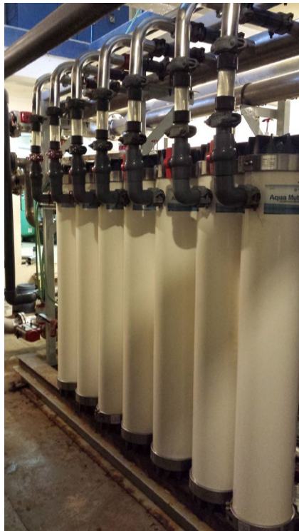
Figure 13. The New Garden City Modules with Rerouted Filtrate Piping
