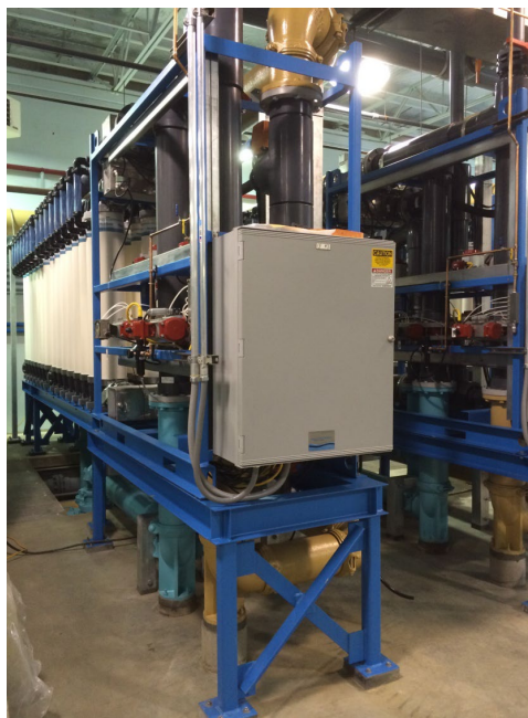
Figure 23. One of the New Byesville Membrane Trains
